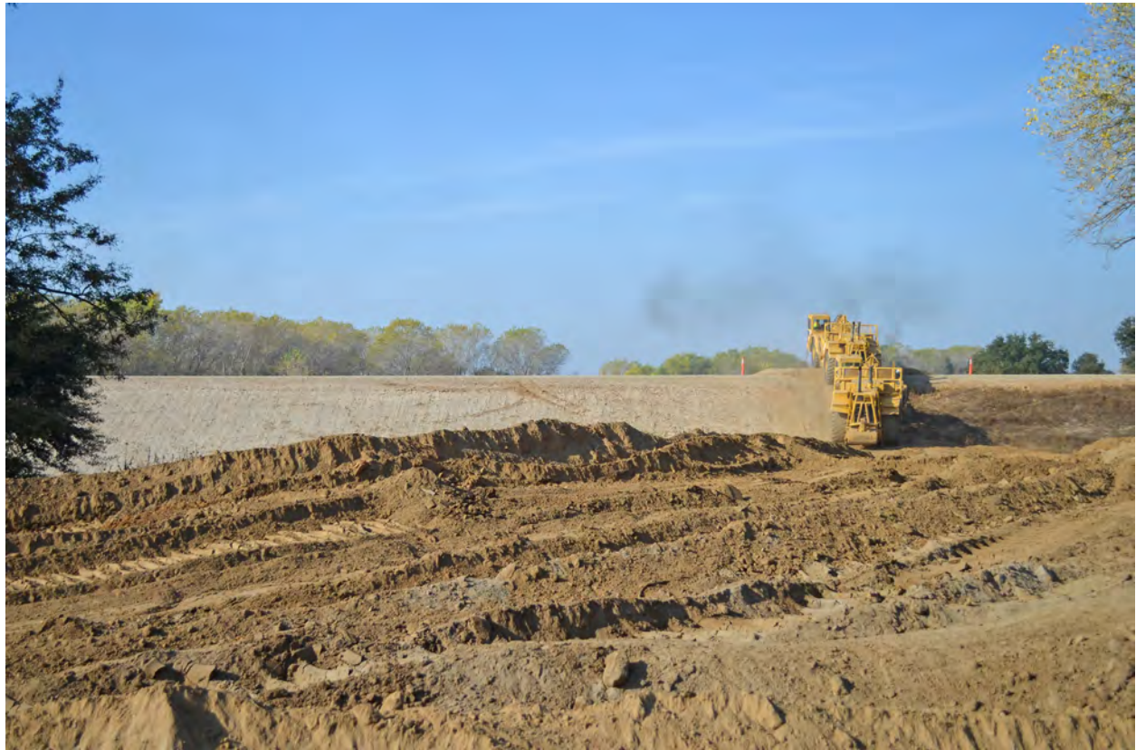
Figure 22.1 Construction equipment traverses a new setback levee to remove material from the old levee along the Sacramento River
